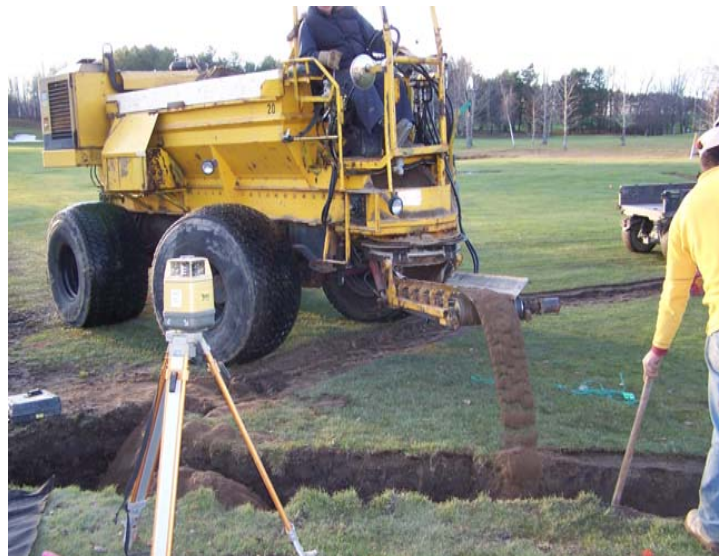
#14 West: This custom built piece of equipment expedites the backfilling of the drainage lines. Photo courtesy of Bob Gaspar
